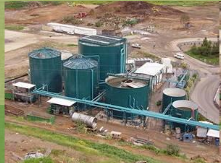
Mechanical biological treatment plant, Tel Aviv, Israel
