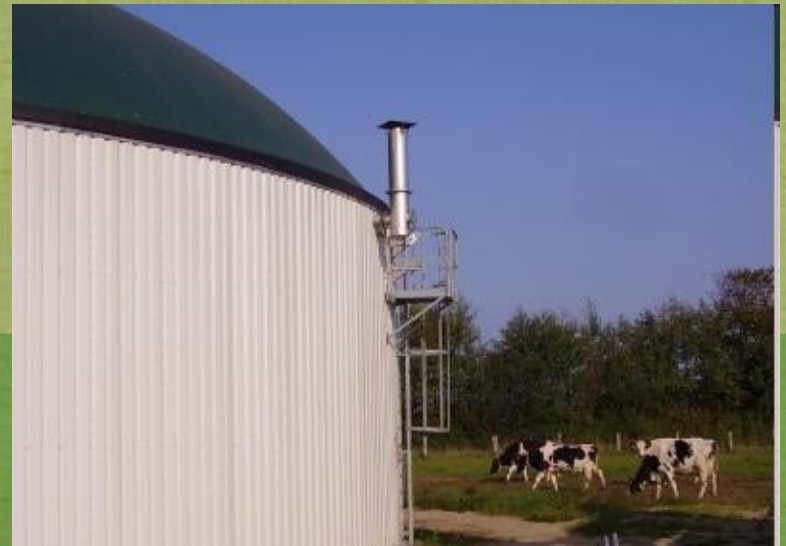
Corn silage digester, Neumunster, Germany
