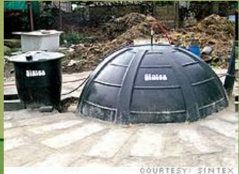
Small scale digester, rural India
