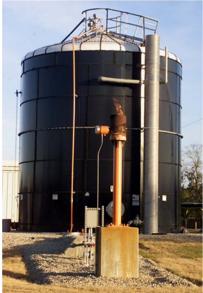
UF/IFAS Fixed-film Anaerobic Digester
